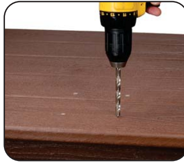
Step 2: Remove post and pre-drill pilot holes to accept 3/8" diameter lag or carriage bolt.
